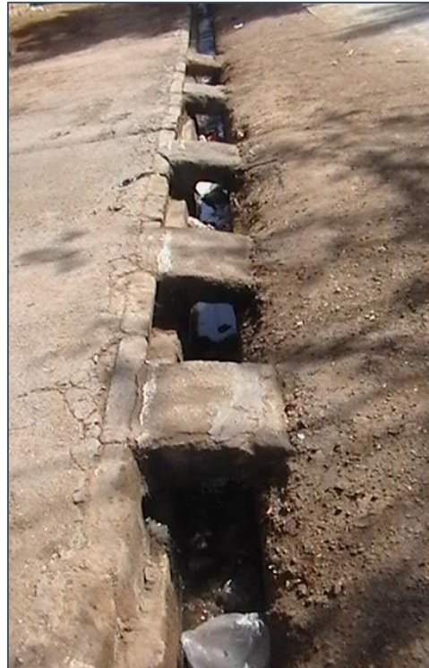
Partially covered drain
